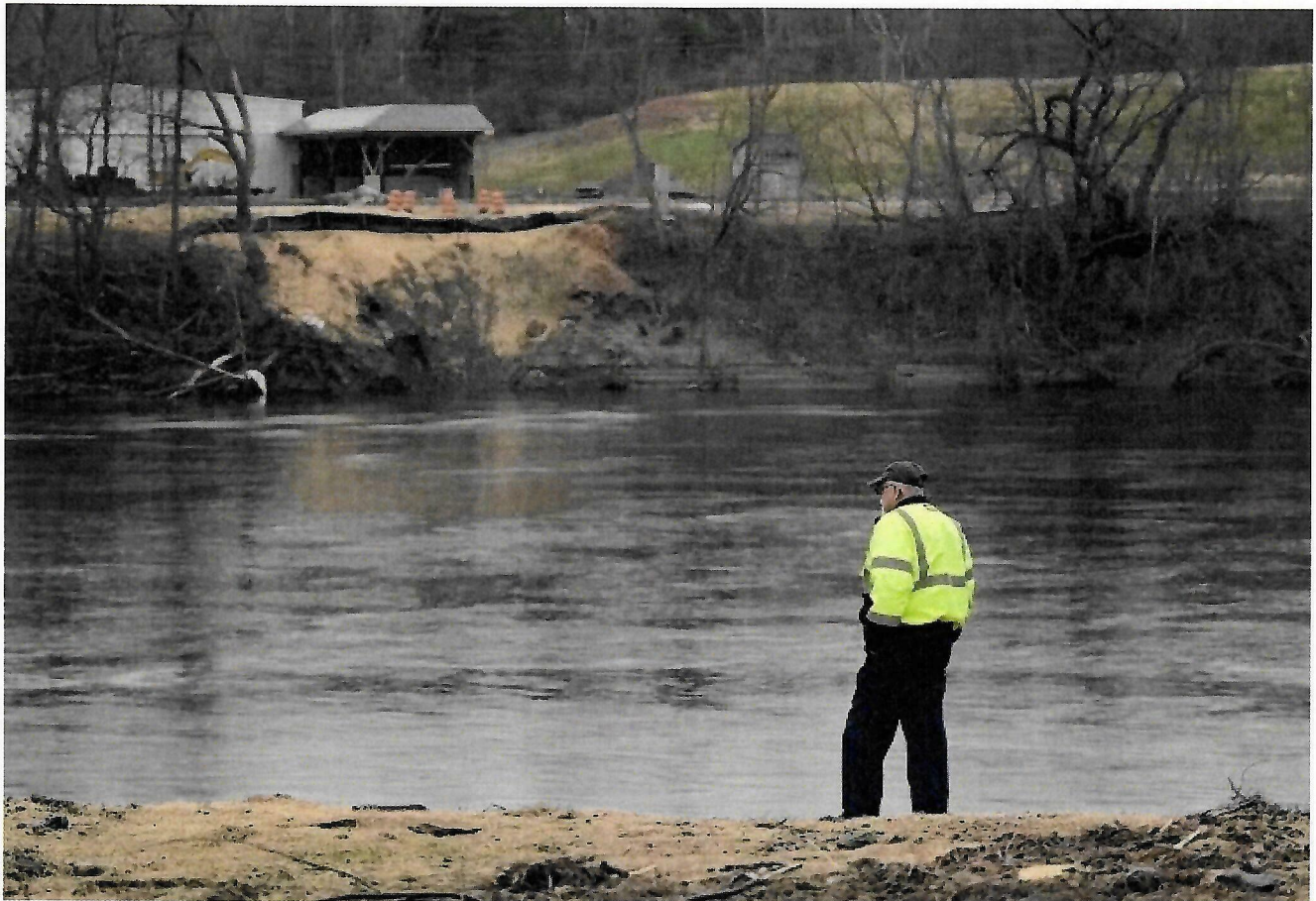
Winslow Public Works Director Paul Fongemie stands on the staging area for piping installation Wednesday at the Chaffee Brook Pumping Station in Winslow. When the project is complete the pipeline will carry sewage under the Kennebec River, from Winslow to Waterville's Kennebec Sanitary Treatment District. Rich Abrahamson/Morning Sentinel
